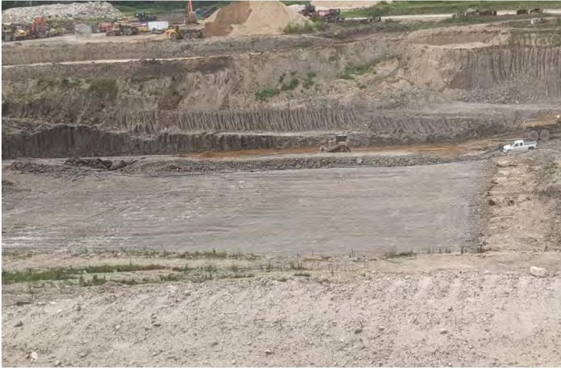
Overview of new cell
