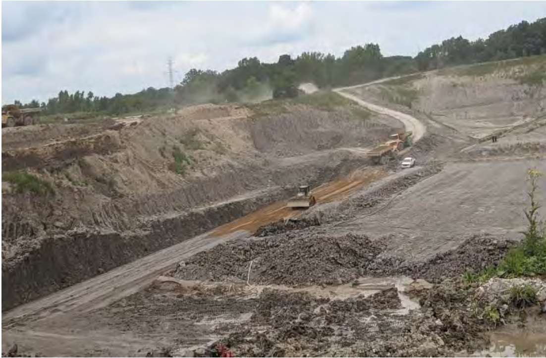
West side of the new cell, construction ongoing, placement of gradient layer
