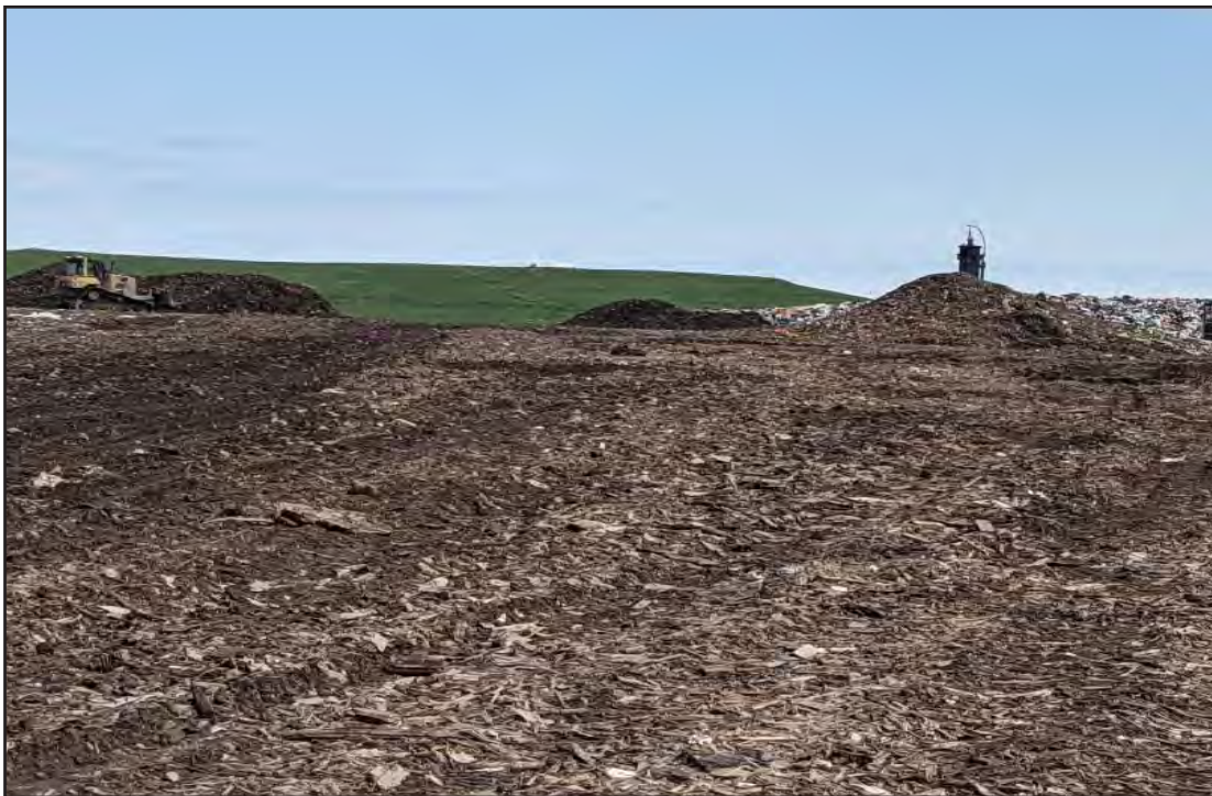
Across top of Phase 7, viewed from the West to the working face
