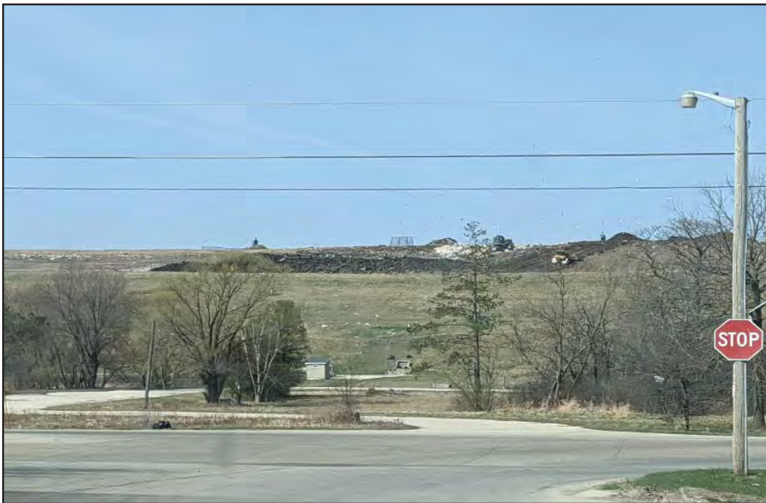
Working face on East slope of Phase 6 bringing up grades before additional placement in Phase 7
