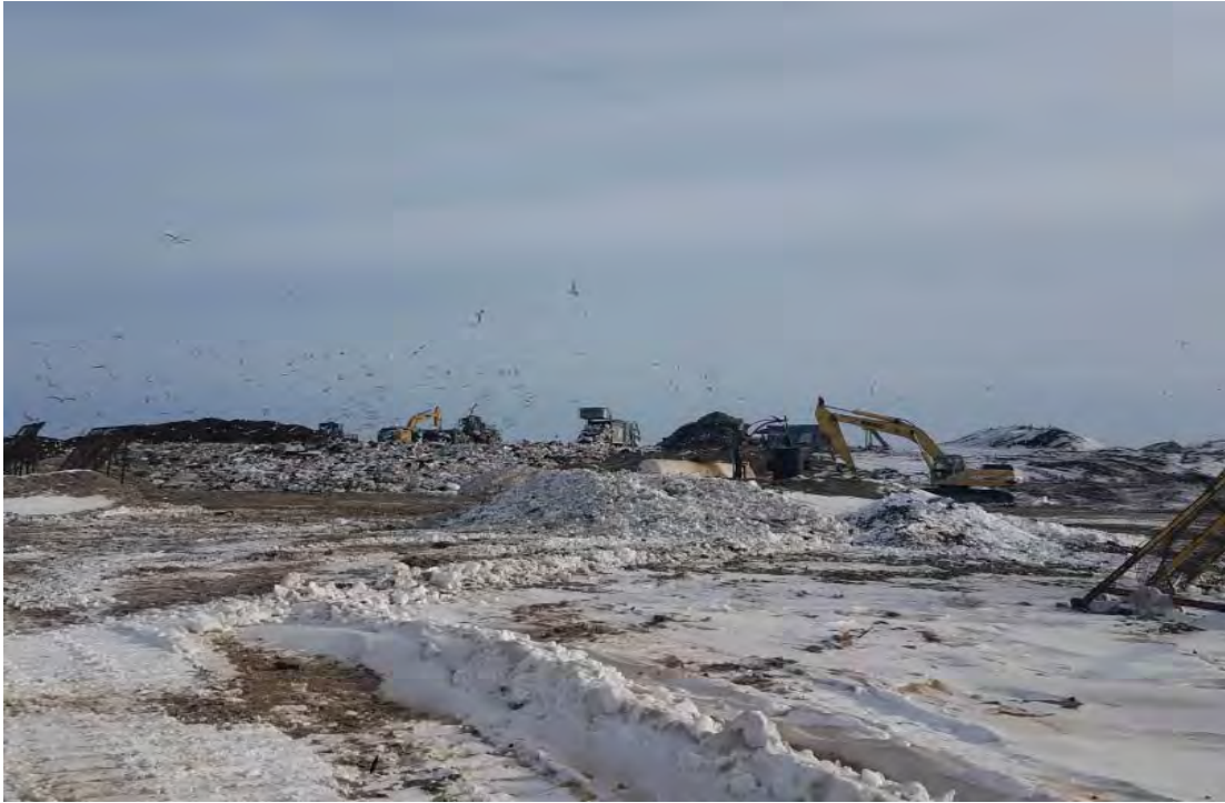
Working face on East edge of Phase 7, completing protective berm development for future tipping
