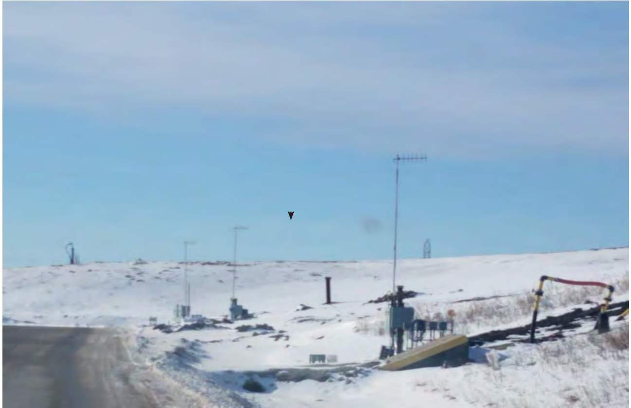
Telemetry antennae on LFG controls about site
