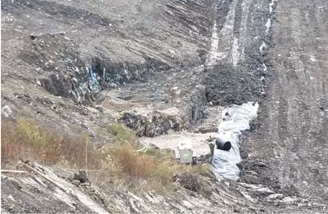
Sump backfilled with stone, more stone will be placed and then cover placed over
