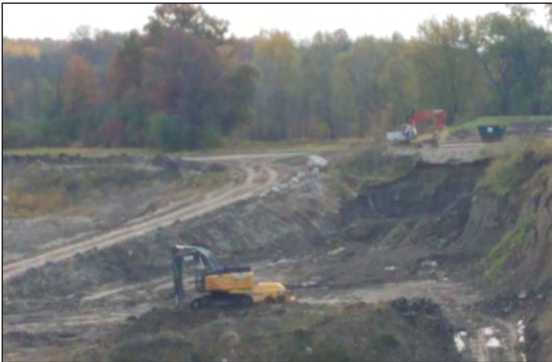
Excavation of soils as needed for construction of road and possibly cover
