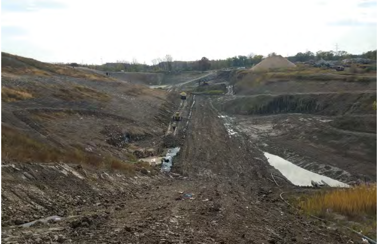
Overview of Phase 7, West edge and temp sed basin, viewed from North
