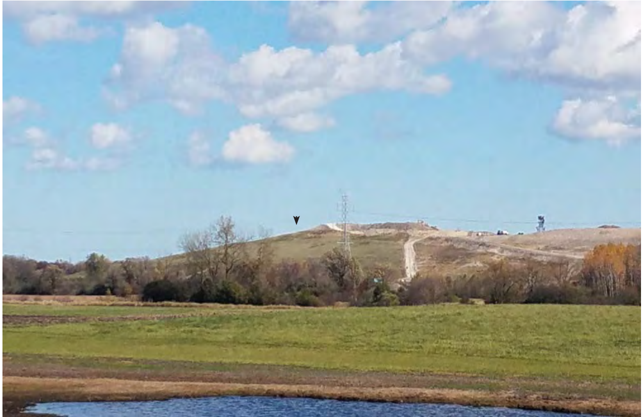
Phase 3, West slope. Erosion from Haul Truck activities.
