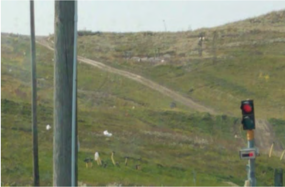
Erosion from the travel of vehicles on the slope of Phase 4
