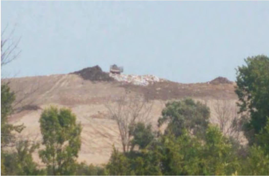
Southwest corner of Phase 7 South, working face being developed to bring lift up to current grade
