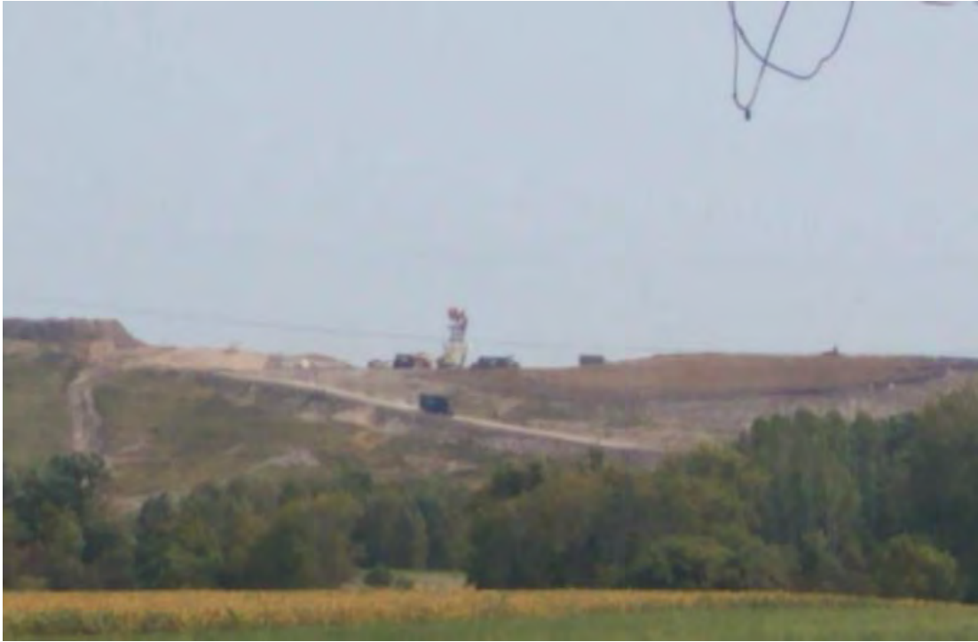
Erosion channels on West slope of Phase 3/7, left side of photo
