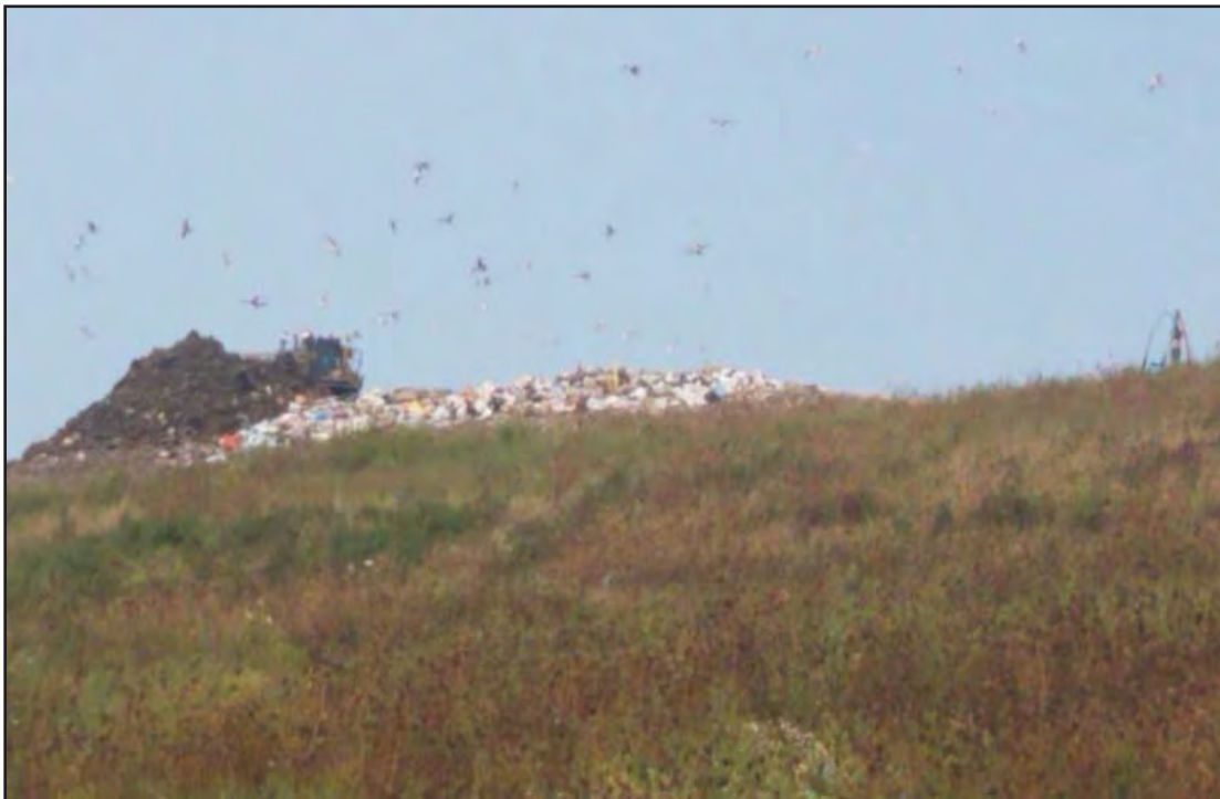
Working face at very South end of Phase 7 South, bring grade up to current lift
