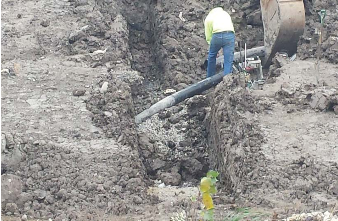
Damaged pipe during drying of clay lift for Closure Area IV
