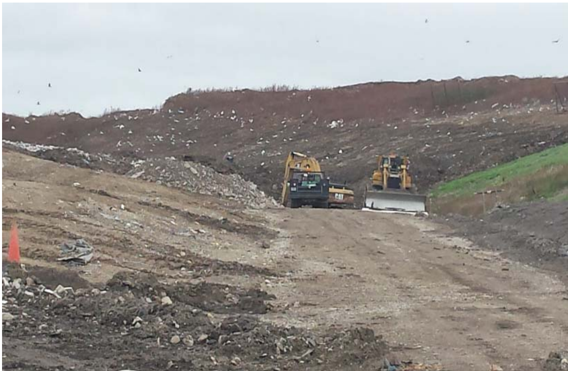
Removal of the access road to Phases 1 thru 3 to allow overlay between Phases 6 and 7
