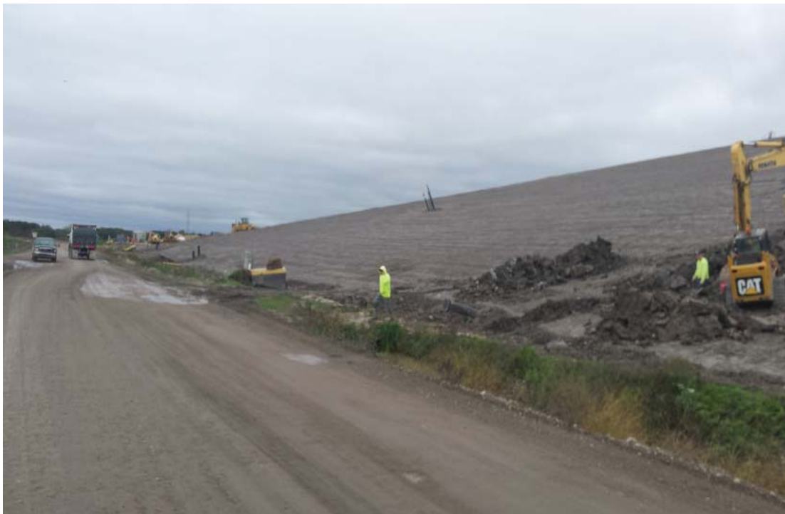
South slope of Phases 5 and 6, closure area IV with first lift of clay placement
