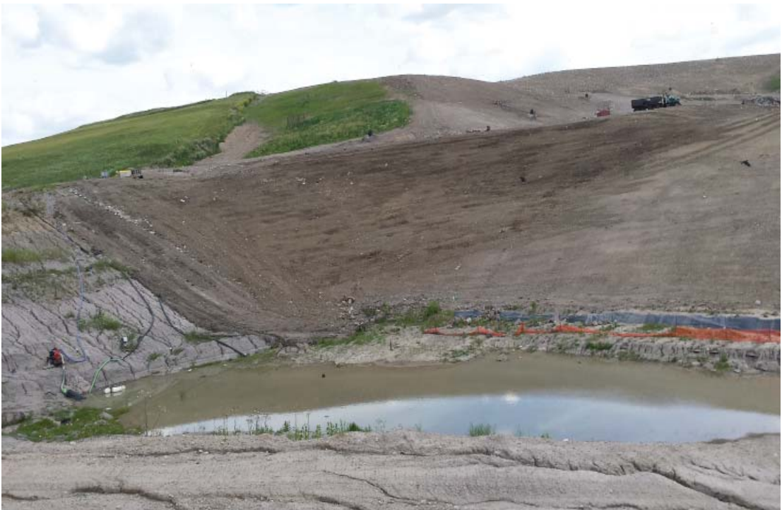
West slope of Phase 7B, waste and cover placement extended out over drainage blanket (stone)
