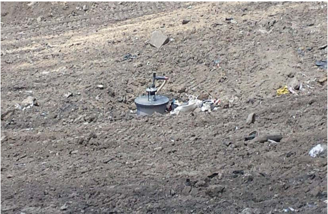
Gas well in Phase 7, requires extension before additional waste can be placed in the area
