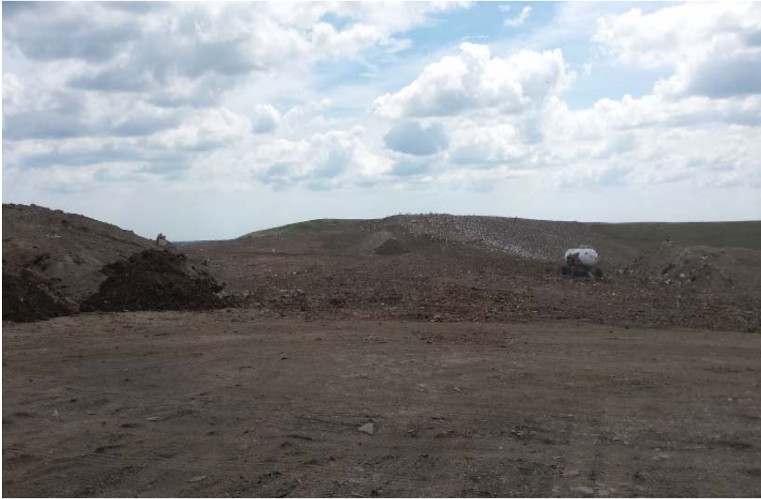
Soil placement over Phase 5/6 trickled to less than one load per day
