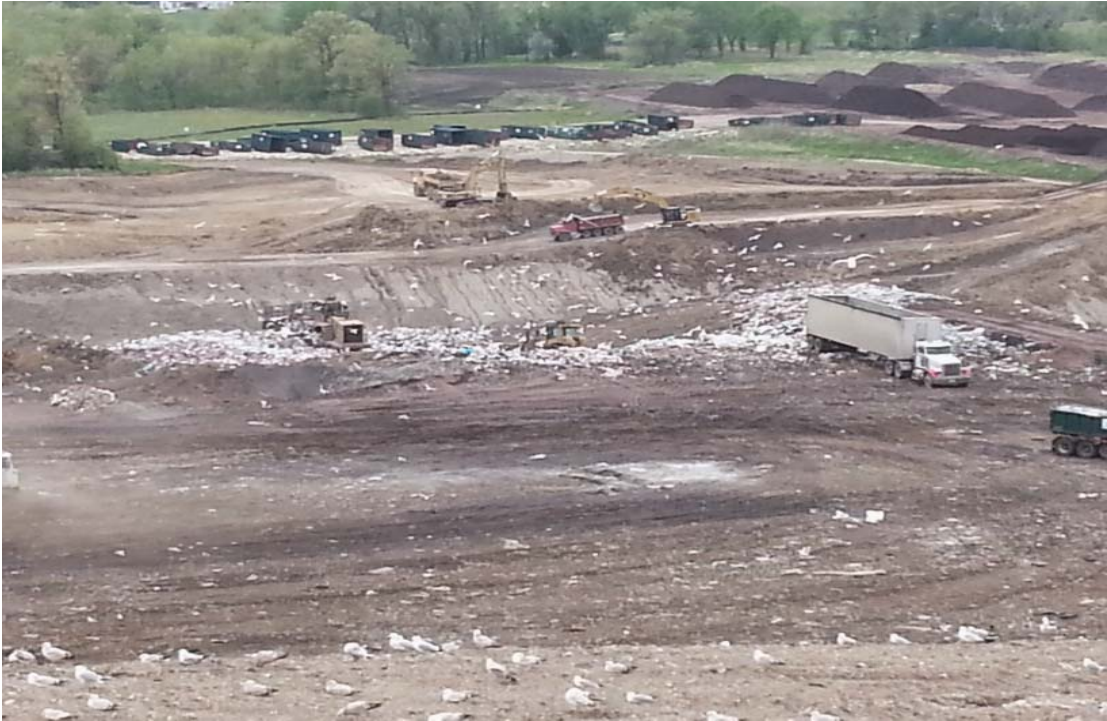
Working face viewed from North, excavation for back haul going on in the background
